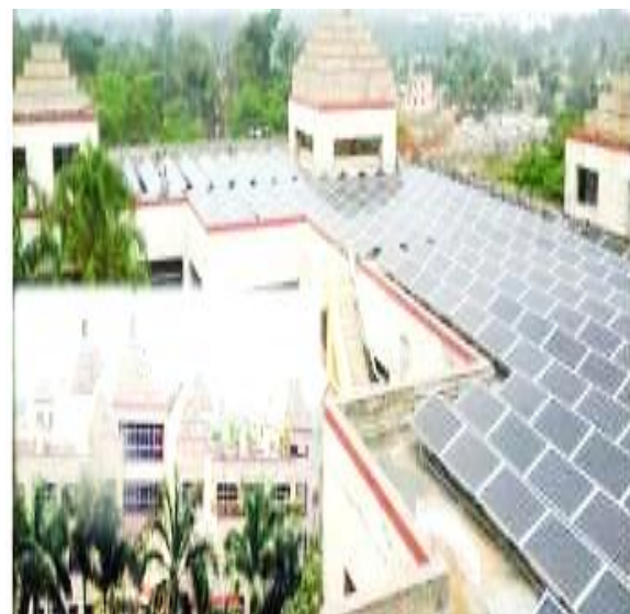
Photo-7.6 Roof Top Solar facility
