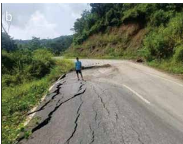
Photo 11.17: Cracks and subsidence in the road along NH-61, Wokha, Nagaland
