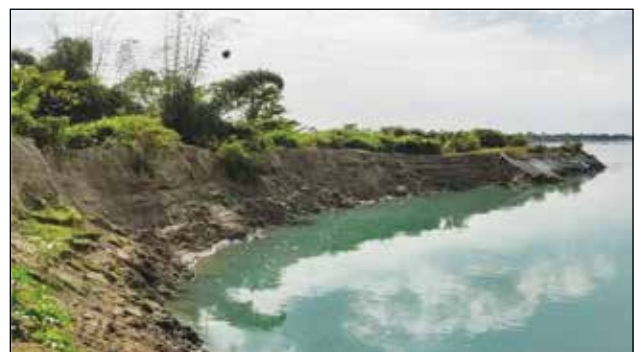
Photo 11.21: Bank erosion along the bank of Brahmaputra at Rohmoriah, Dibrugarh District, Assam.
