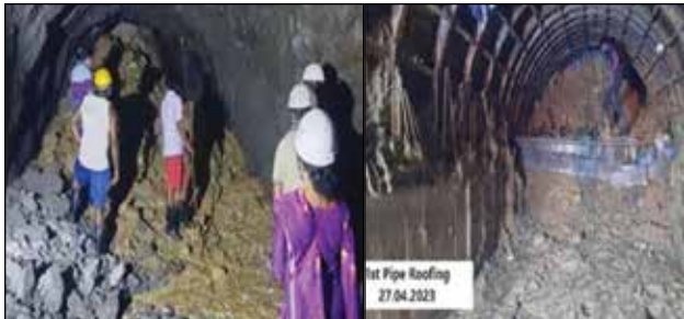
Plate 1: 1 st Collapse from face-IV, ingress of debris flow on 7 th January 2023
