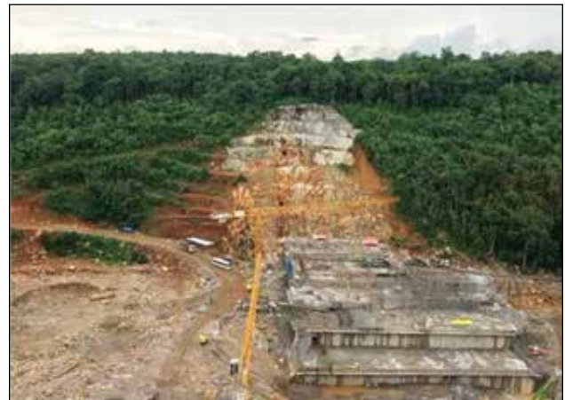
Phot 11.16: View of different dam blocks under construction on the left Abutment, Kopili Hydroelectric Project (110MW).
