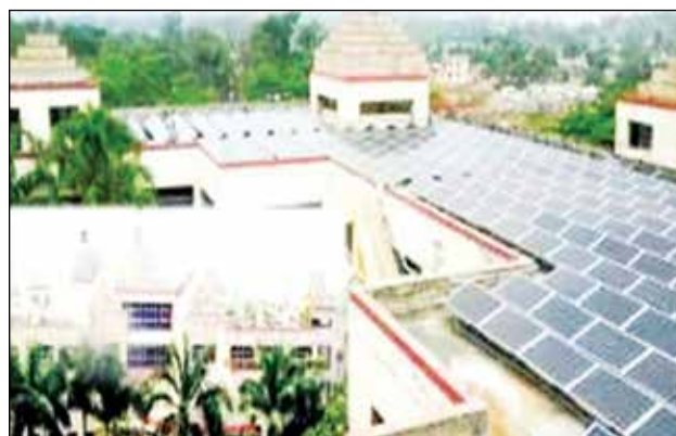
Photo-7.7 Roof Top Solar facility
