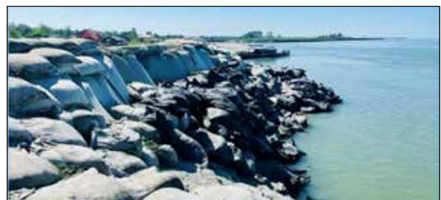
Photo 11.22: Collapse of Geobags due to toe erosion along the bank of Brahmaputra River at Rohmoriah, Dibrugarh District, Assam
