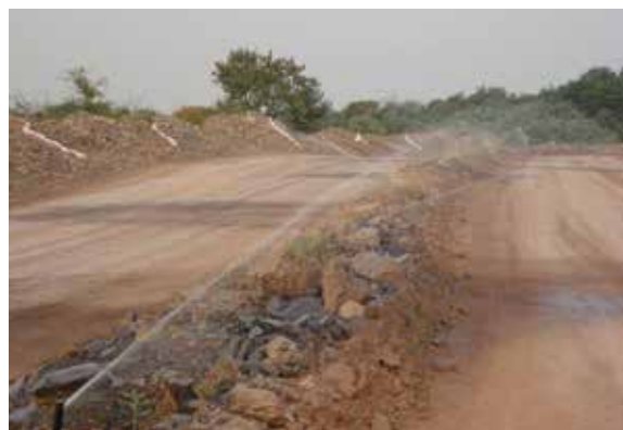
Automatic Water Sprinklers on Road
