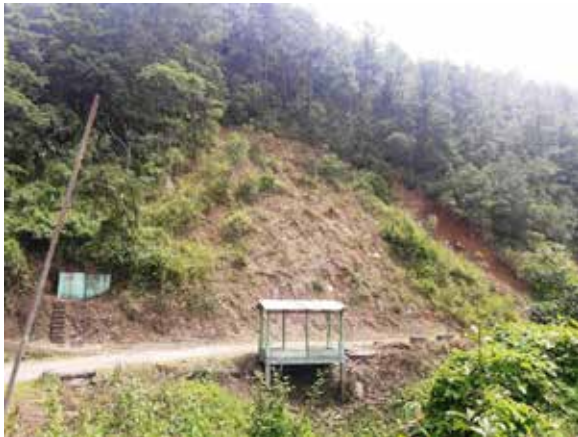
Debris slide about 1.5km North of Sailulah Village on East Lungdar-Sailulah PMGSY road, Mizoram
