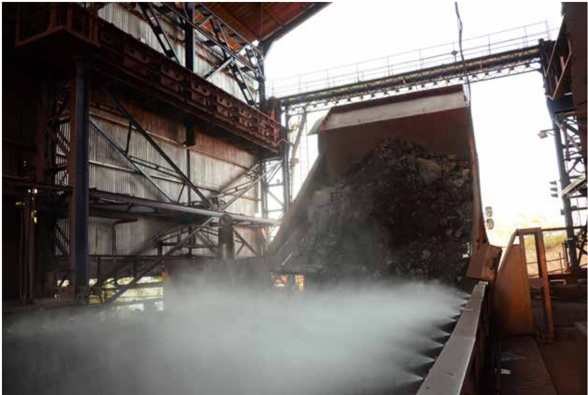
Dry Fog system in Ore crusher feeding point
