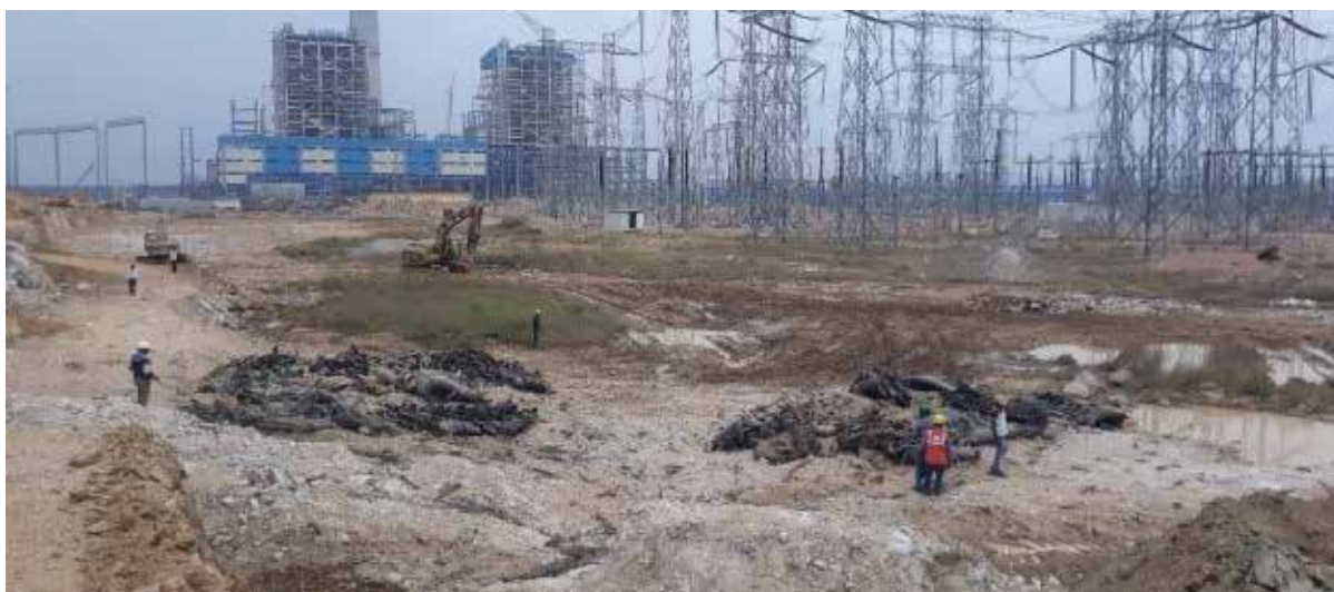
Fig. 1: Safe excavation of around 3.5 lacs m 3 of hard rock by controlled blasting for the Darlipalli Super Thermal Power Project, Stage-I, NTPC
