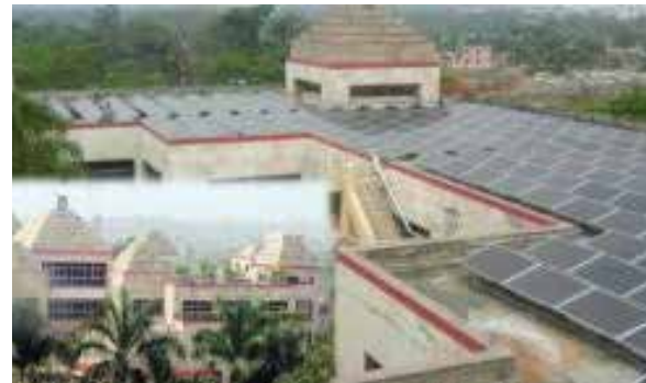
Rooftop Solar Panels
