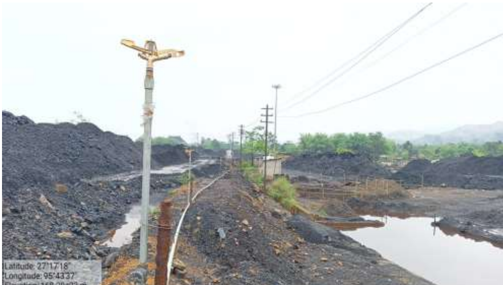
Water Sprinklers for Dust Suppression
