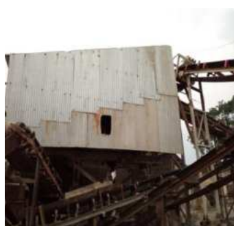
COVERED CRUSHING UNIT
