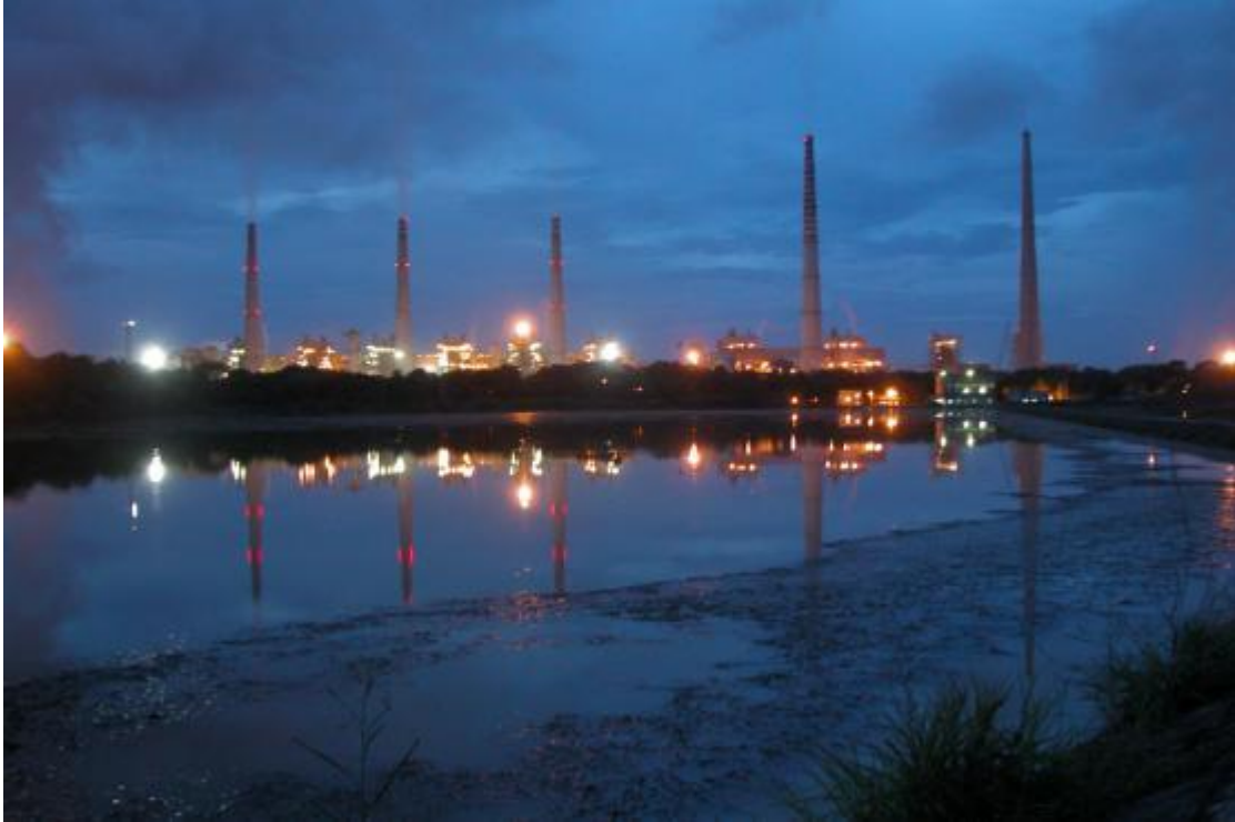
Figure 6 : Captive Power Plant, Angul
