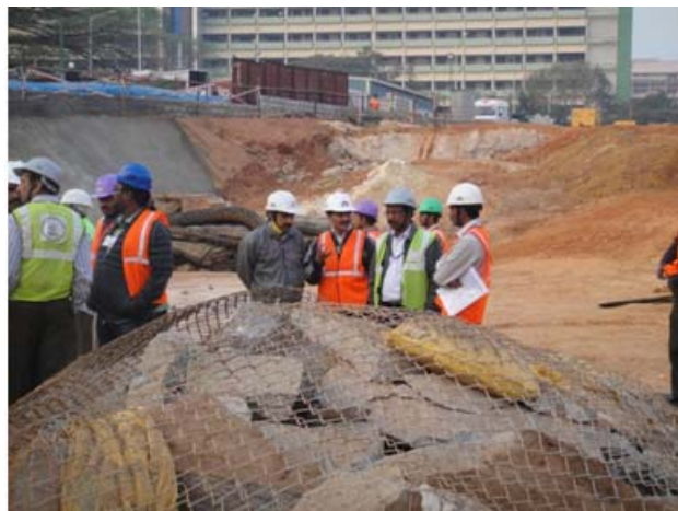
Demonstration of wedge cut blast and control of fly rock for metro project, Bangalore
